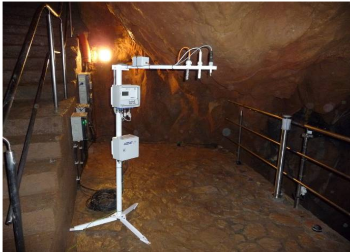
Fixed Monitoring Station with Sensors and Data Logger
